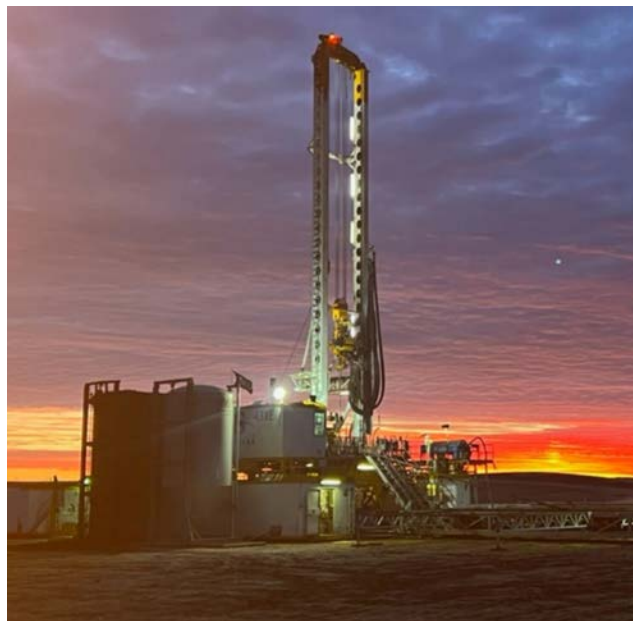
Beautiful sunrise at the Savanna 431 drilling rig on the Saturn 10-20-25-17W3 oil well location. This is the first section of land to be drilled on what Saturn said was its transformational Viking Acquisition that closed July 6, 2022.
