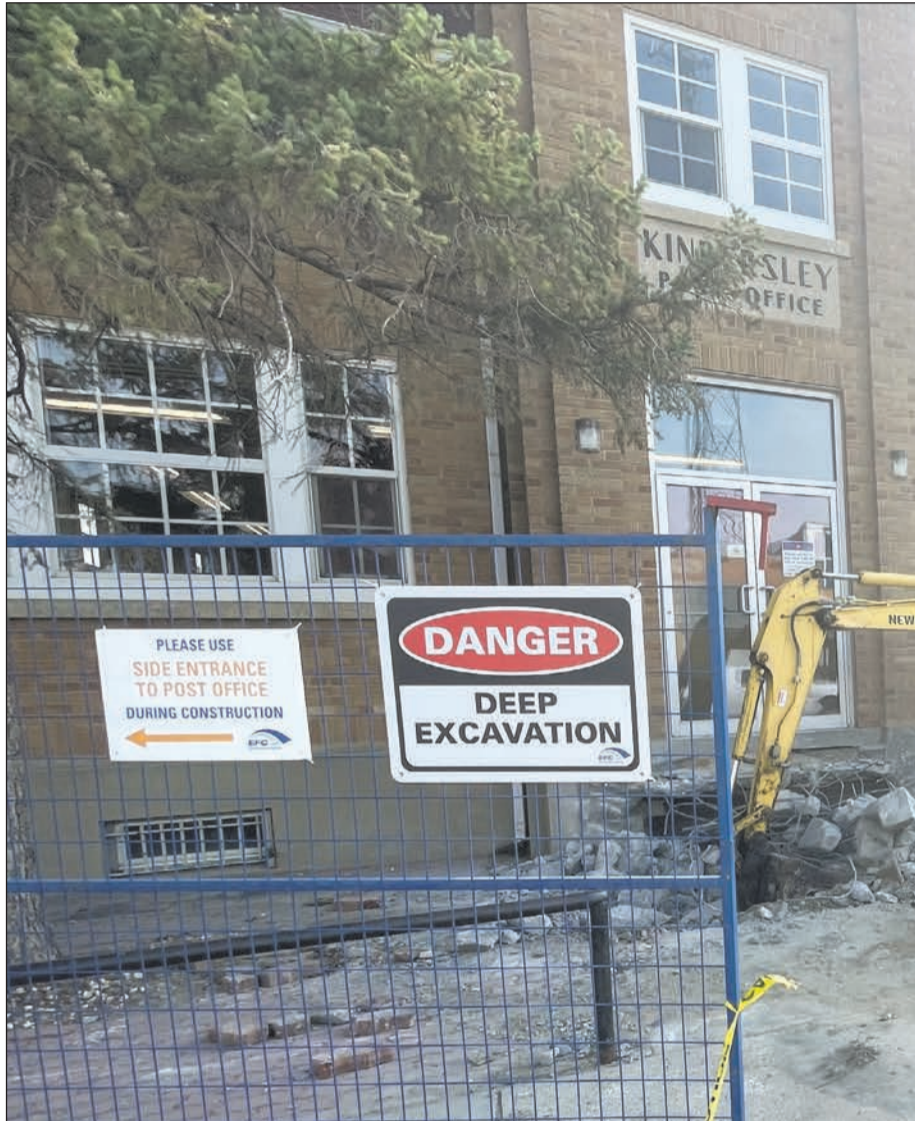
Crew removed the concrete steps in the front of the Kindersley Post Office. PHOTO BY JOAN JANZEN
