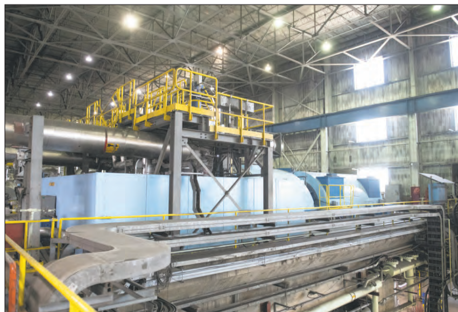
Boundary Dam Unit 3 turbine and generator. PHOTO BY BRIAN ZINCHUK
