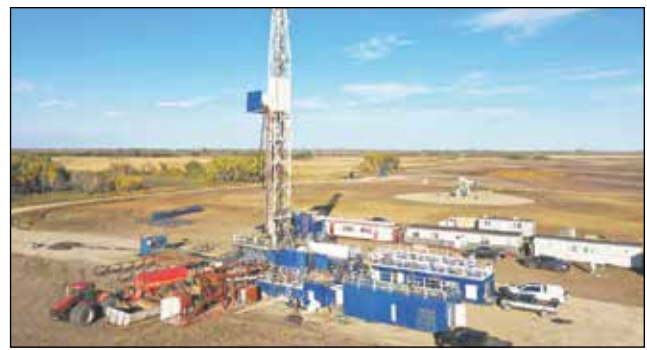
Alliance Drilling Rig 2 was drilling northeast of Glen Ewen on gorgeous Sept. 29. Despite weather that has been very agreeable most of the fall, many oil companies are cutting back on their drilling programs. PHOTO BY BRIAN ZINCHUK
