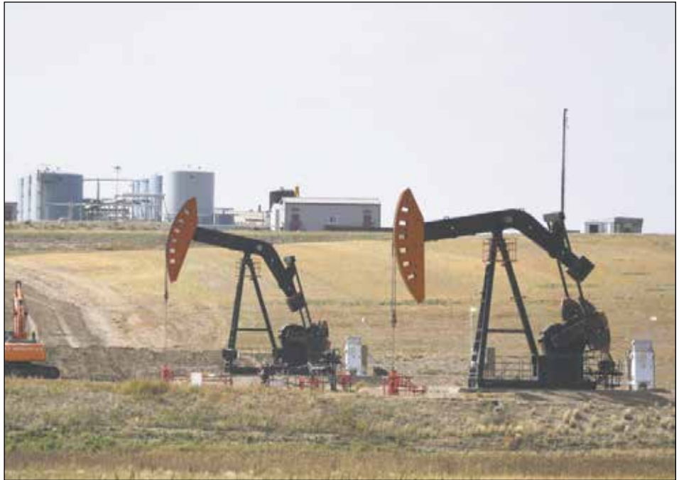
Pumpjacks near a battery southwest of Torquay, Saskatchewan. PHOTO BY BRIAN ZINCHUK
