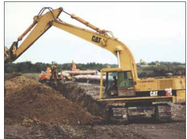
Construction near Moosomin in 1997 of the pipeline that was supposed to eventually become the Energy East pipeline. Of the 4600 kilometres for the whole route, 3000 are already in the ground, as seen here. Photo by Brian Zinchuk, who was a worker on the project.
