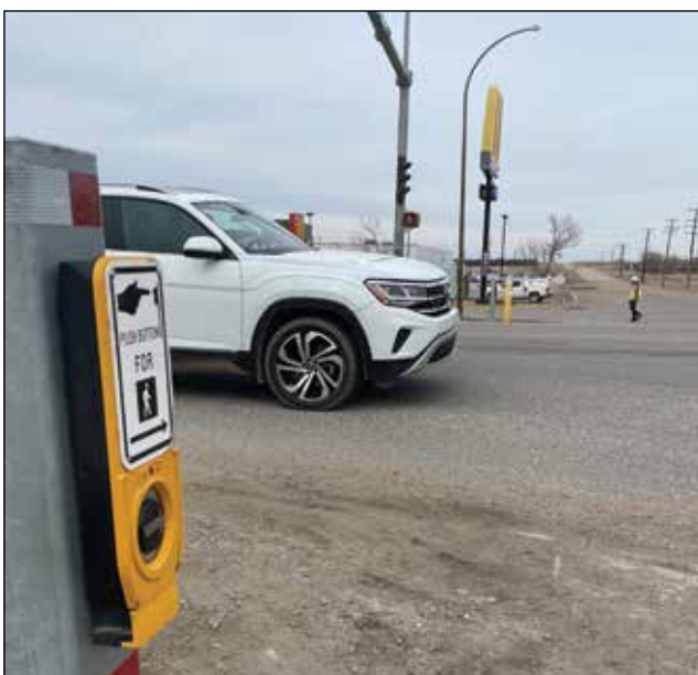
The intersection at Ditson Drive will receive new traffic lights and pedestrian light improvements. Construction will begin in May, 2024. PHOTO BY JOAN JANZEN
