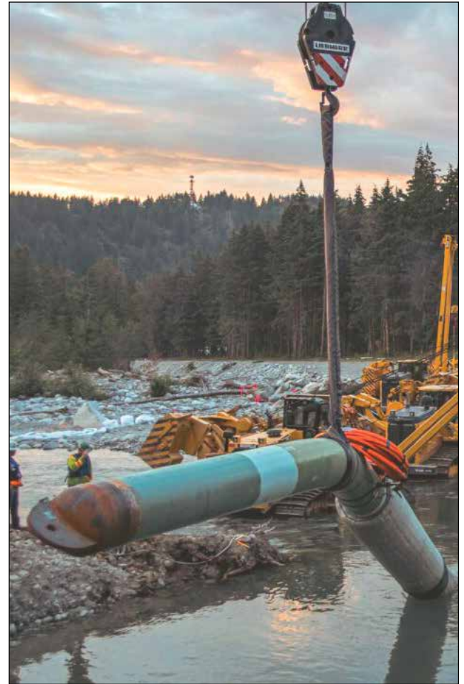
In August, 2022, Trans Mountain recently completed installation of new pipeline and the replacement of an existing segment under the Coquihalla River. The work was done simultaneously to minimize impact to the environment and neighbours. LINKEDIN/TRANS MOUNTAIN
