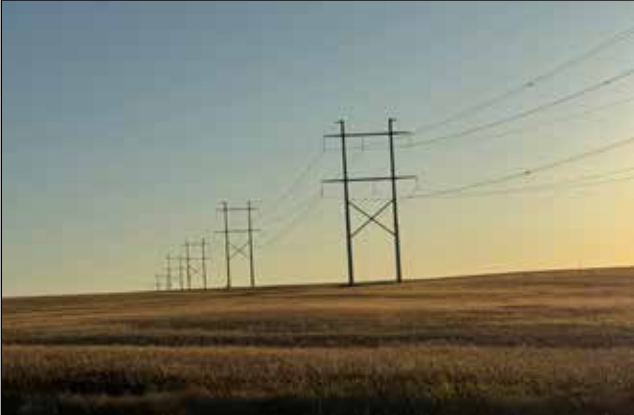
This power transmission line north of Swift Current eventually leads to the McNeill Station intertie.
