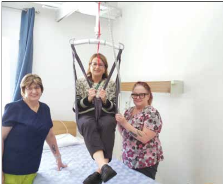
Lifting care forward: Eston Health Centre facility manager Jocelyn Irvine, assisted by staff members Mona Antony, left, and Chris Mazzei, demonstrates one of two newly installed wall and ceiling lifts. The equipment was donated by the Dr. David S. Mulder Eston and District Health Foundation Inc.
