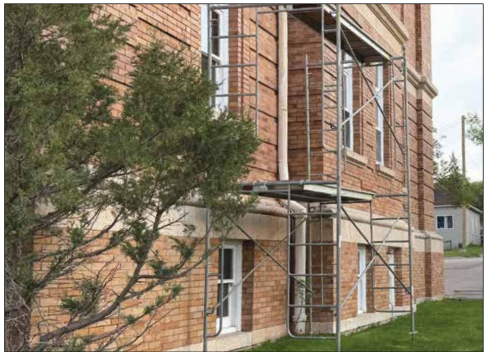
Scaffolding set up around Kerrobert's courthouse right now involves Rocco Stone Masonry from Saskatoon repointing areas of the exterior bricks that have lost mortar. PHOTO COURTESY VERONICA SMITH
