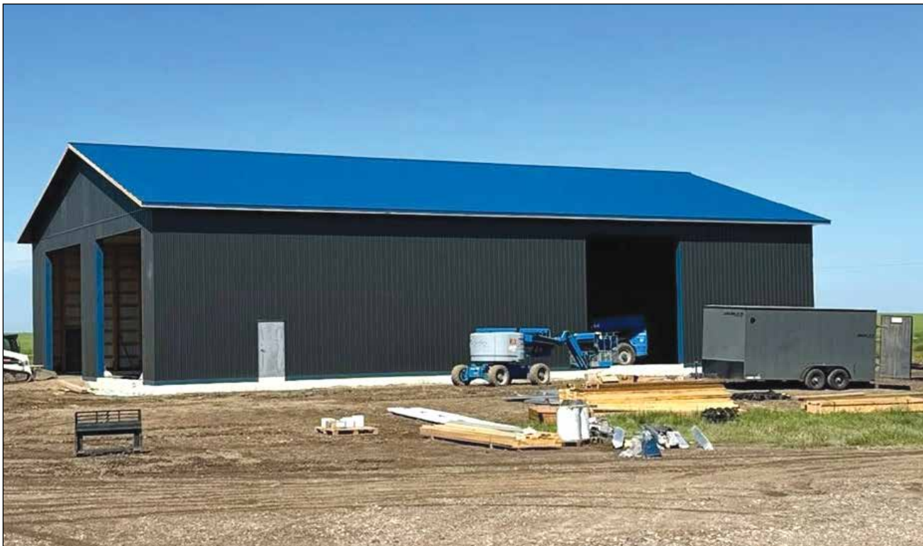
NEW SHOP TAKES SHAPE. Construction of the R.M. of Mariposa's new Public Works shop was well underway in August 2025. The municipality will host an official grand opening and public open house July 24, giving residents an opportunity to tour the facility. PHOTO COURTESY R.M. OF MARIPOSA FACEBOOK PAGE.
